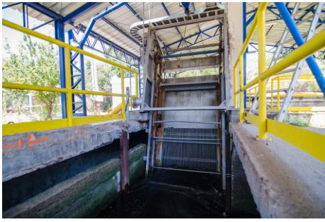
View of the automatic sorting grille
