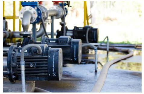
Pressure pumps to clean the filter
